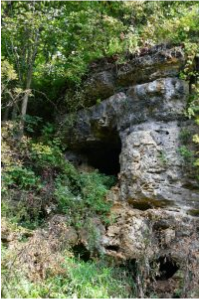
Another hole in the wall
